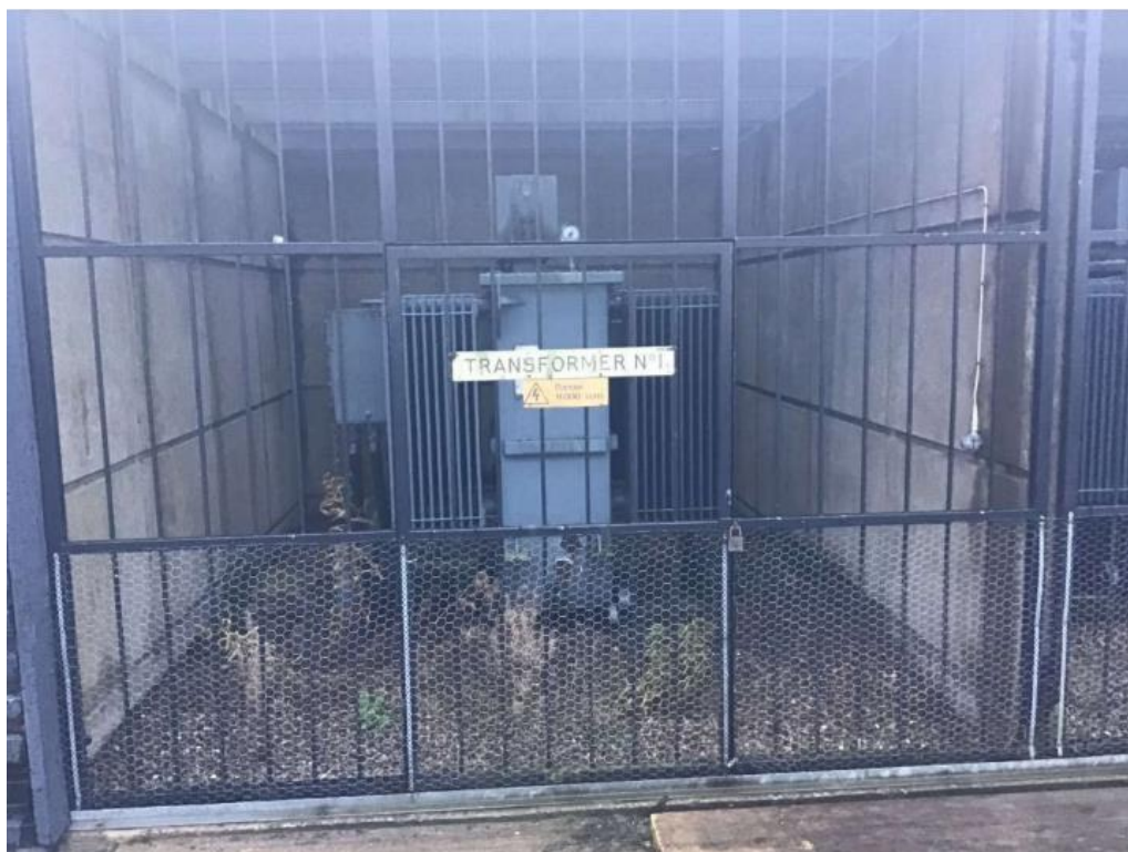
Figure 7 Plant 1 T1 transformer 1 currently isolated
