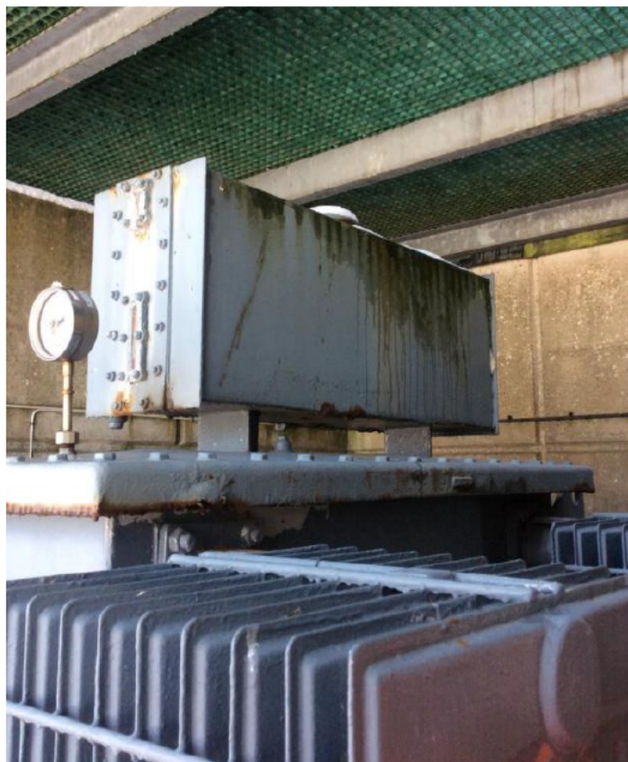
Figure 9 Leaking oil from conservator tank and corrosion
